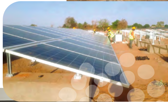
Solar power plant in Burkina Faso
