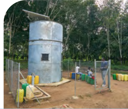
Solar-powered water distribution point: water tower and solar pumping system
