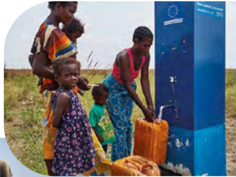
Automatic Solar Standpipe
